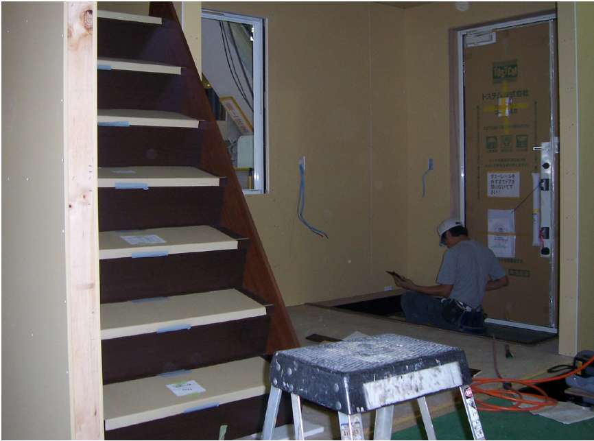
Figure 4.6 Offline module (customized stairs take a lot of labor that varies with choices).
